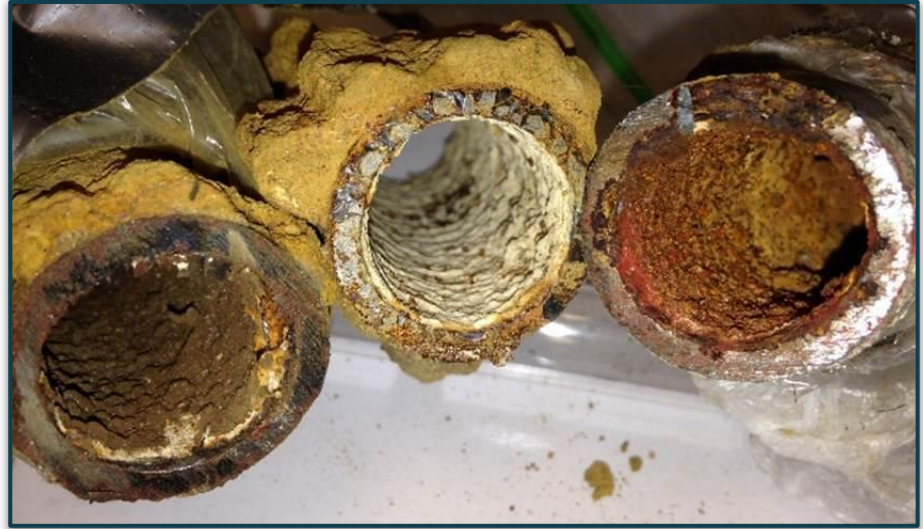
Decaying sewage pipes and septic systems contaminate water and give rise to leakages
